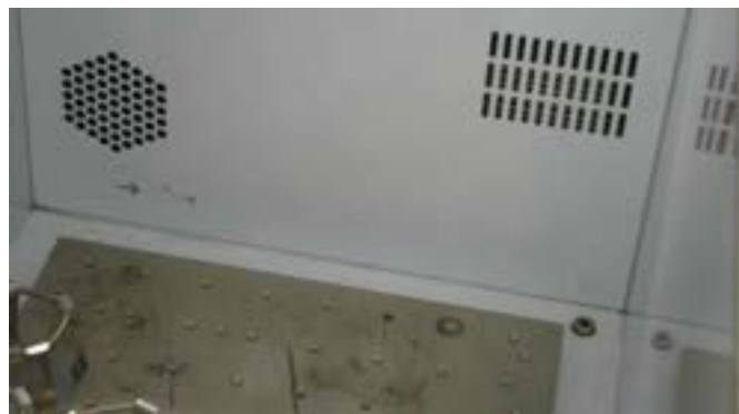
Chamber Heater Circulation Passages
